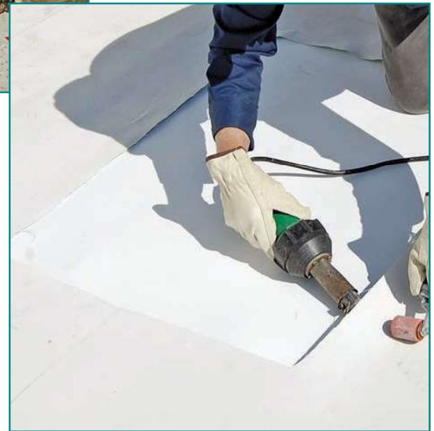
Figure 12 – Repair of aged TPO membrane with a new patch welded to the aged core. Image courtesy of WSRCA.
