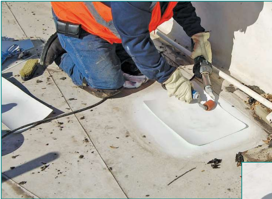
Figure 11 – Repair of aged TPO membrane with a new patch welded to the aged cap. Image courtesy of WSRCA.
